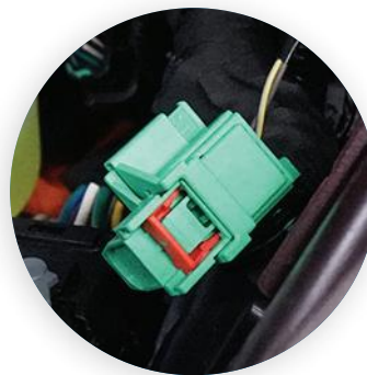
The Low Voltage Service Disconnect should be restored to the ON position and red locking tab pressed down to secure the circuit.
